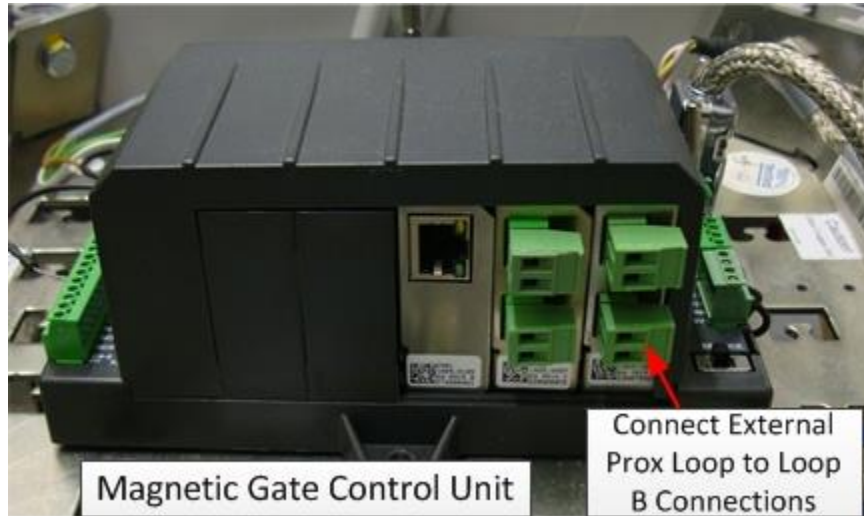
Figure 28. Magnetic Gate Control Unit
